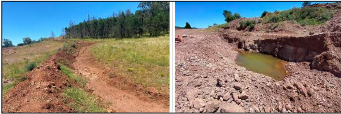
Figure 11: Left: stormwater diversion bund and Figure 12: Right: sediment basin/sump (source: EIS)
